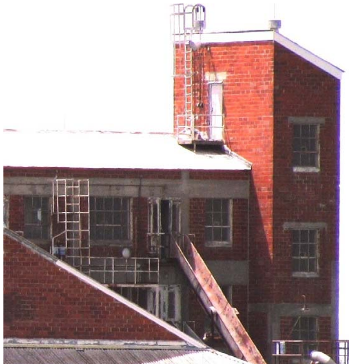
The 900 Area's three-story melt tower and emergency evacuation slide will no longer puncture the skyline one decontaminated and demotion are complete.
